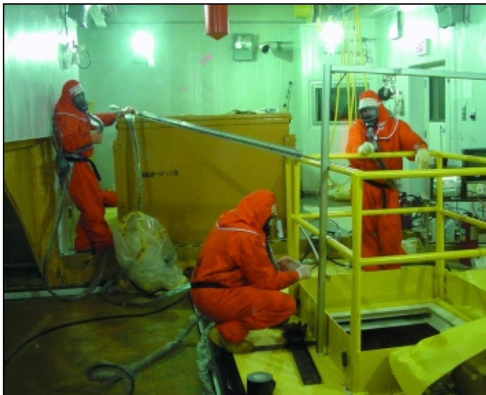
D&D operators don flame-retardant suits and prepare to insert the 13-ft torch through the rolling hatch and down into the crane room below for cutting.
