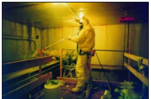
A D&D operator sprays a fixative coating on the failed crane equipment planned for size-reduction at West Valley. The coating helps to minimize airborne contamination.
